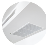
Ducted heating and cooling system
